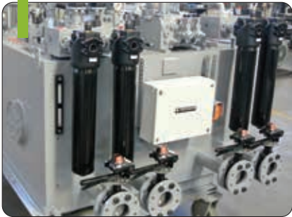
Main engine driven power unit hydraulic tank.
