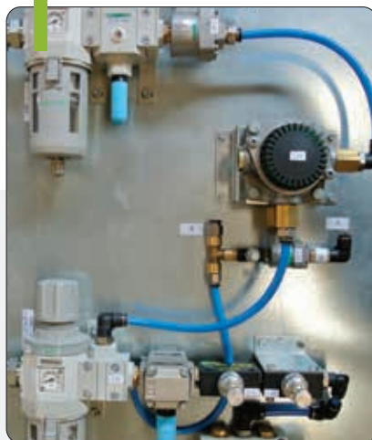
Winch pneumatic control panel
