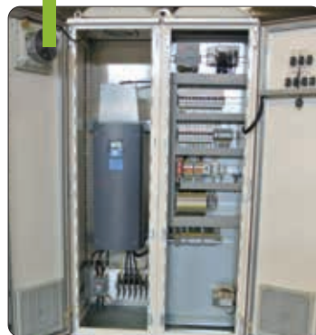
Winch control cabinet with frequency converter
