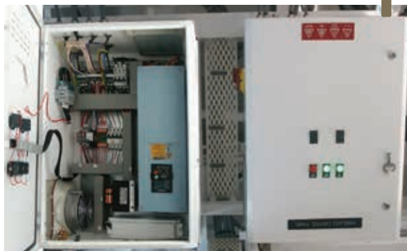
Windlass control panels with frequency converters
